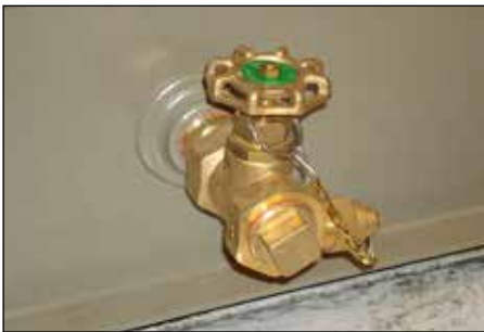
Figure 3. Drain valve with sampler.
