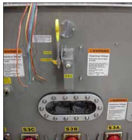
Figure 8. VFI transformer with visible break.
